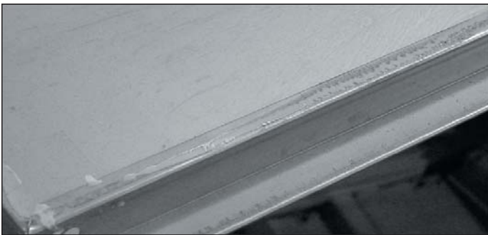
Failure mode – incorrect repositioning methods
