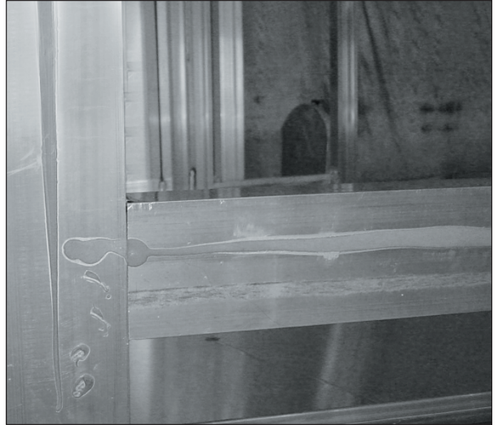
Failure mode – coating changes
