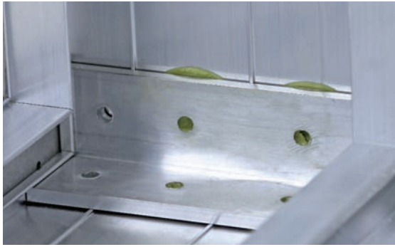
Figure 1 An adhesively bonded plate created a joint that protects the end of the bracket from peel loads.
